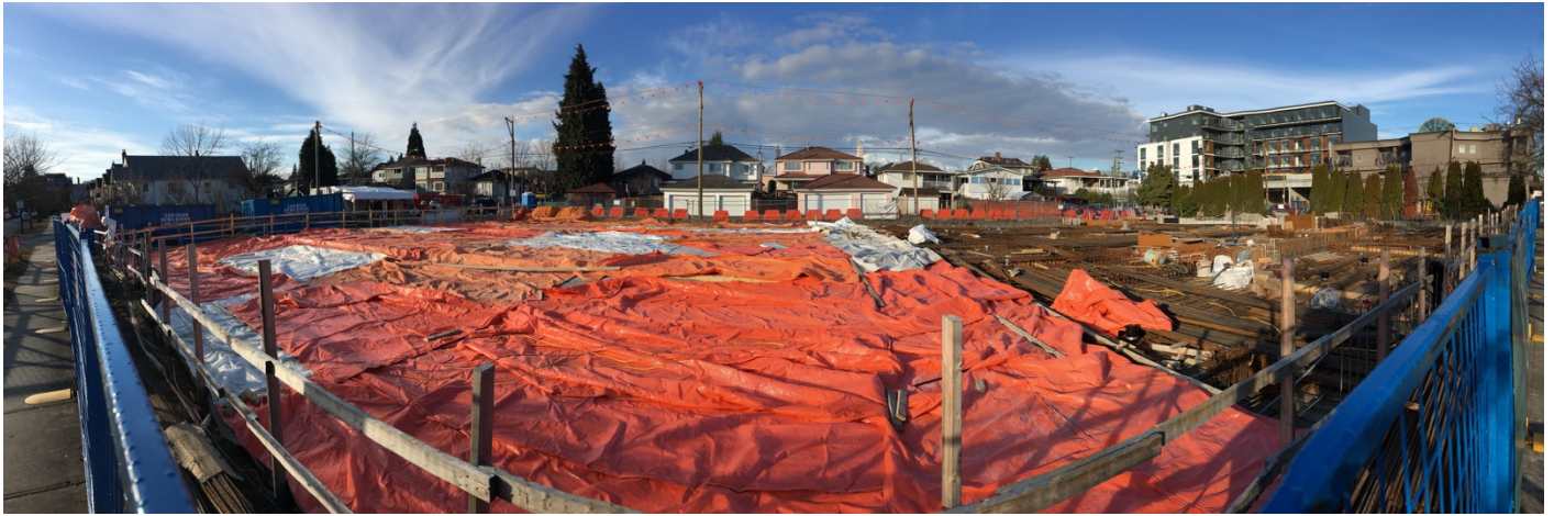
Picture 7: The first half of the concrete suspended slab under the plastic cover (March 01, 2019)
